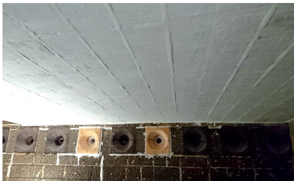
Fig. 8 Finished roof, Superwool® XT stack modules with PCW blanket fold in between
