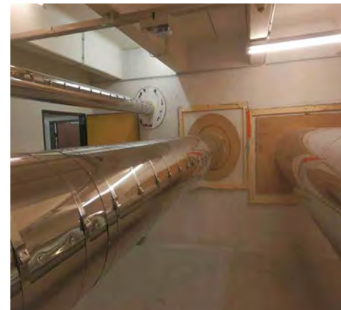
Typical test arrangement of pipes tested insulated with the FireMaster pipe fire protection system
