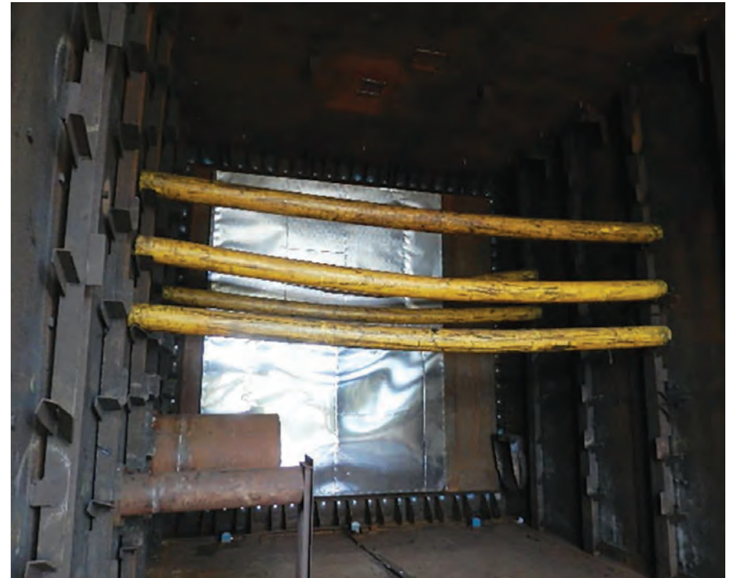
FireMaster vessel system installed on back wall of explosion chamber prior to explosion testing.
