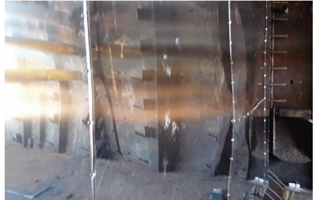
FireMaster Vessel system after 2nd explosion test. No damage occurred to the cladding. An inspection of the insulation was made after removal of the cladding and no damage or compression of the insulation thickness was noted.
